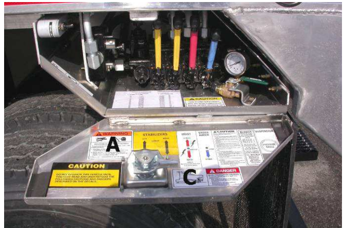
Fig. 3-4 Control Box Trailer (Typ)
