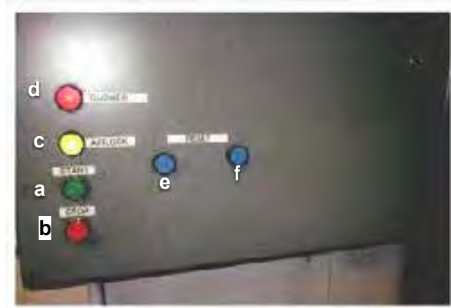
FIG. 2 MASTER CONTROL PANEL
