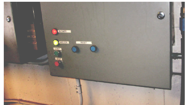
Master Control Panel
